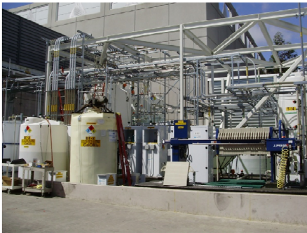
Shown: FRS-6000-2500-3-6FP-T-AX-4-N4XS-FL 2500 gallon triple tank sequencing batch fluoride removal system with equalization tank (not shown) with chemical day tanks, and a 460 VAC PLC based system.
