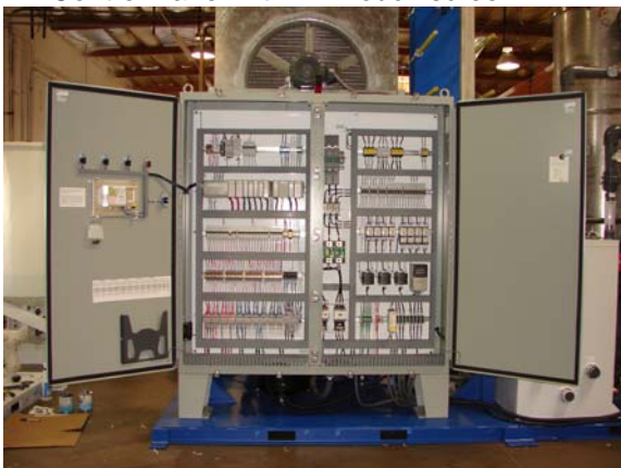
Control Panel with AB Touch screen HMI
